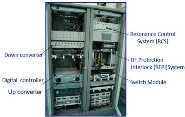
Fig.8: Integrated RF control system commissioned at HTS, RRCAT.
