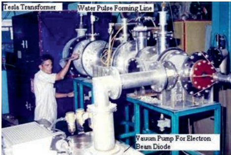
Figure 1.1. KALI-1000 pulse power system.
