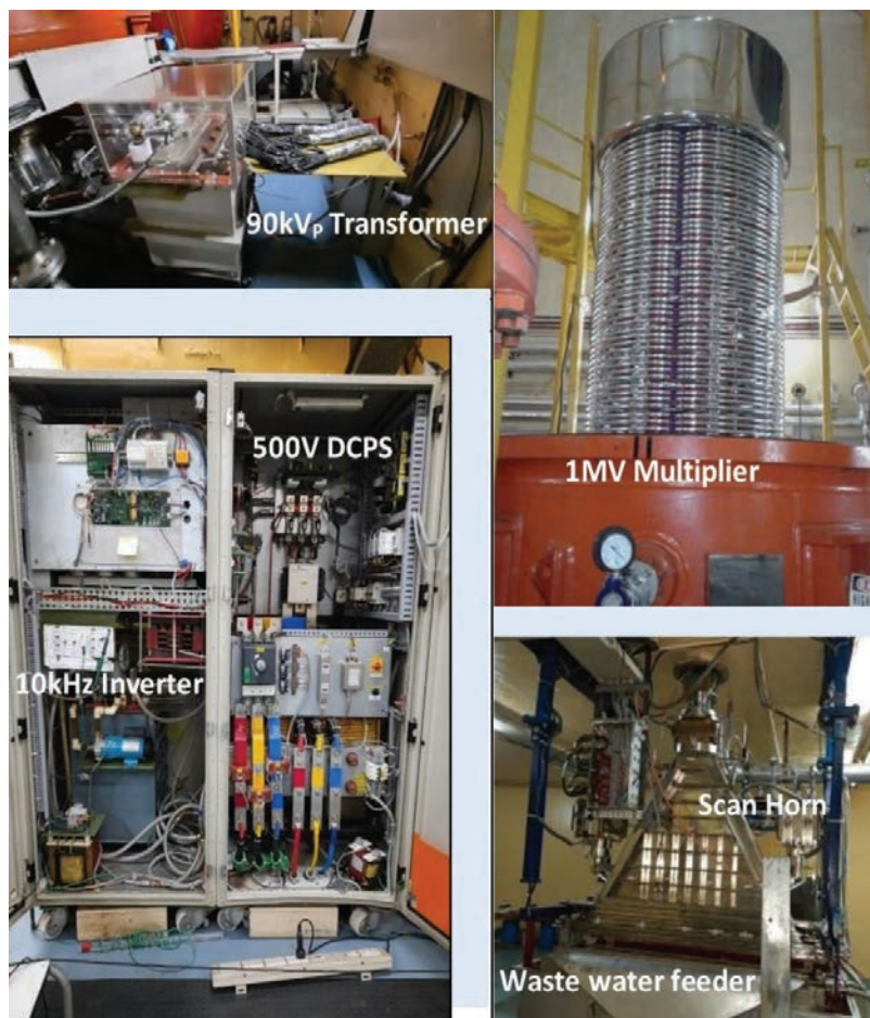
Figure 11.2: Subsystems and waste water treatment set up of 1 MeV DC accelerator.
